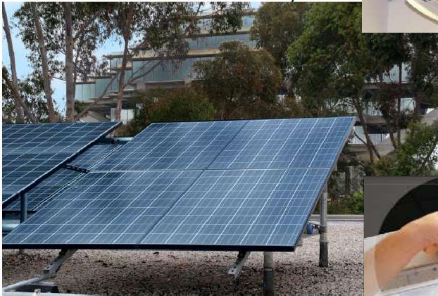
DC Source: Dedicated Solar Array
