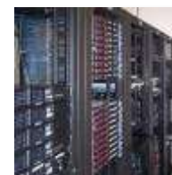
Data & Telecom Centers
