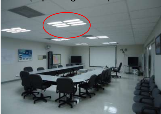
2x4 60W Troffer (replacing 160W)
