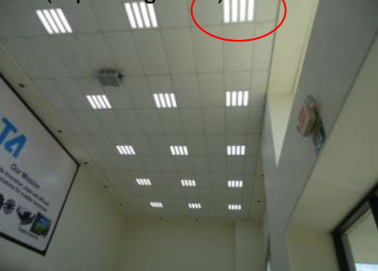
2x2 40W Troffer (replacing 80W)
