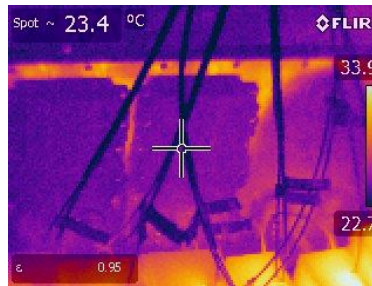
Thermal data of the Medium Voltage Bridge of DAB Converter System
