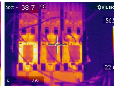
Thermal data of the Low Voltage Front End Converter System
