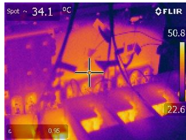
Thermal data of the Medium Voltage Front End Converter System
