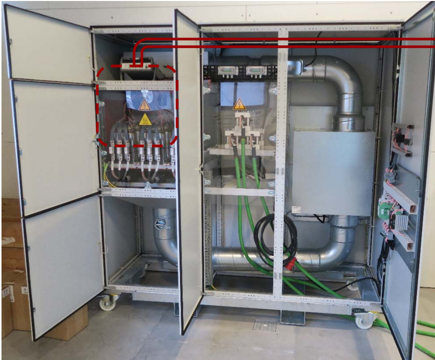
Capacitor bank testing setup at Aalborg University
